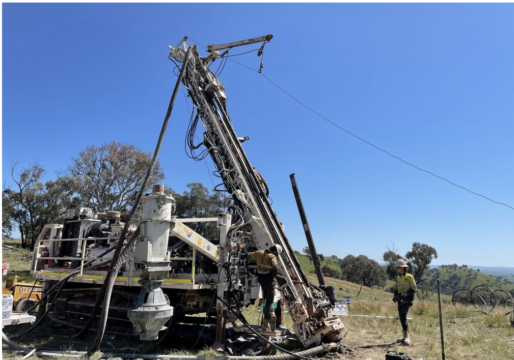
Image 1: RC 650 track mounted drill rig onsite at the Emu prospect located in EL8586, Gundagai North
