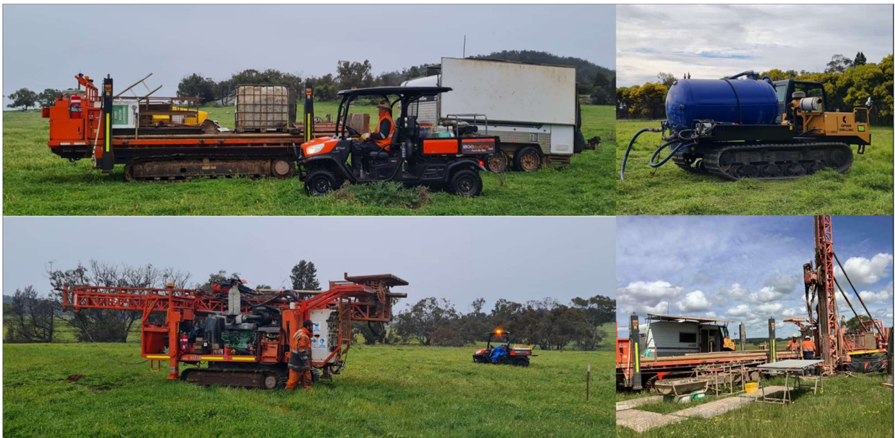
Image one: Ongoing diamond core drilling at Narraburra, clockwise from top left, track mounted rod slew towing support equipment, track mounted sump vacuum, drill rig site setup and tramping of track mounted drill rig to drill hole location.
